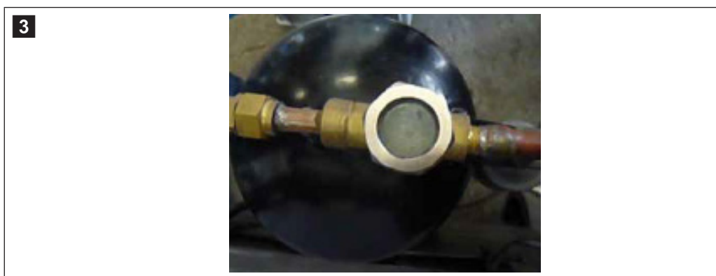
Fig. 3: Sight glass from the flushing tank of the A/C service station
